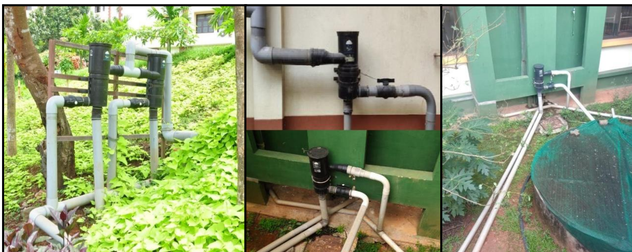
Roof rainwater harvesting units for recharging borewells and for open wells in Yenepoya (Deemed to be University), Mangalore, Karnataka
