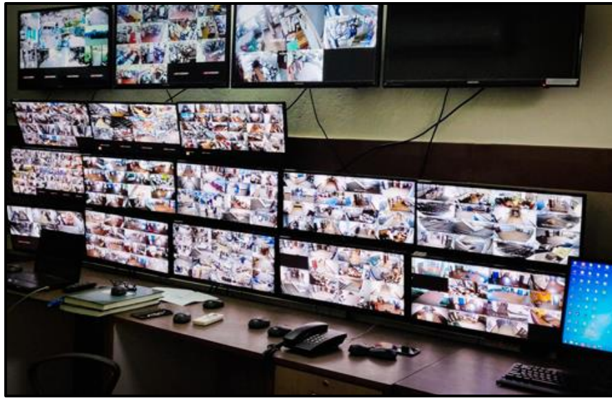
Safety measures - CCTV Monitoring Activities in Yenepoya (Deemed to be University), Mangalore, Karnataka
