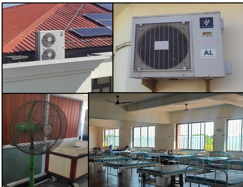
Ventilation Facilities in Yenepoya (Deemed to be University) Buildings
