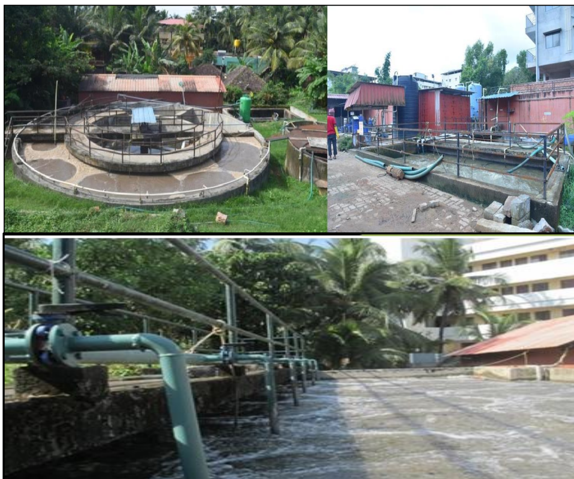
Sewage Treatment Plant (STP) Unit in Yenepoya (Deemed to be University), Mangalore, Karnataka
