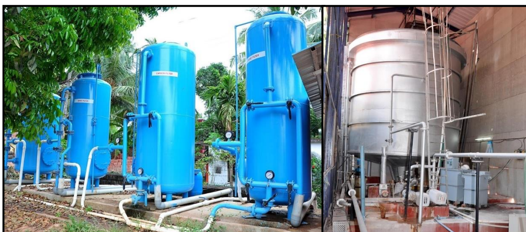
Water Treatment plant and Effluent treatment plant in Yenepoya (Deemed to be University), Mangalore, Karnataka
