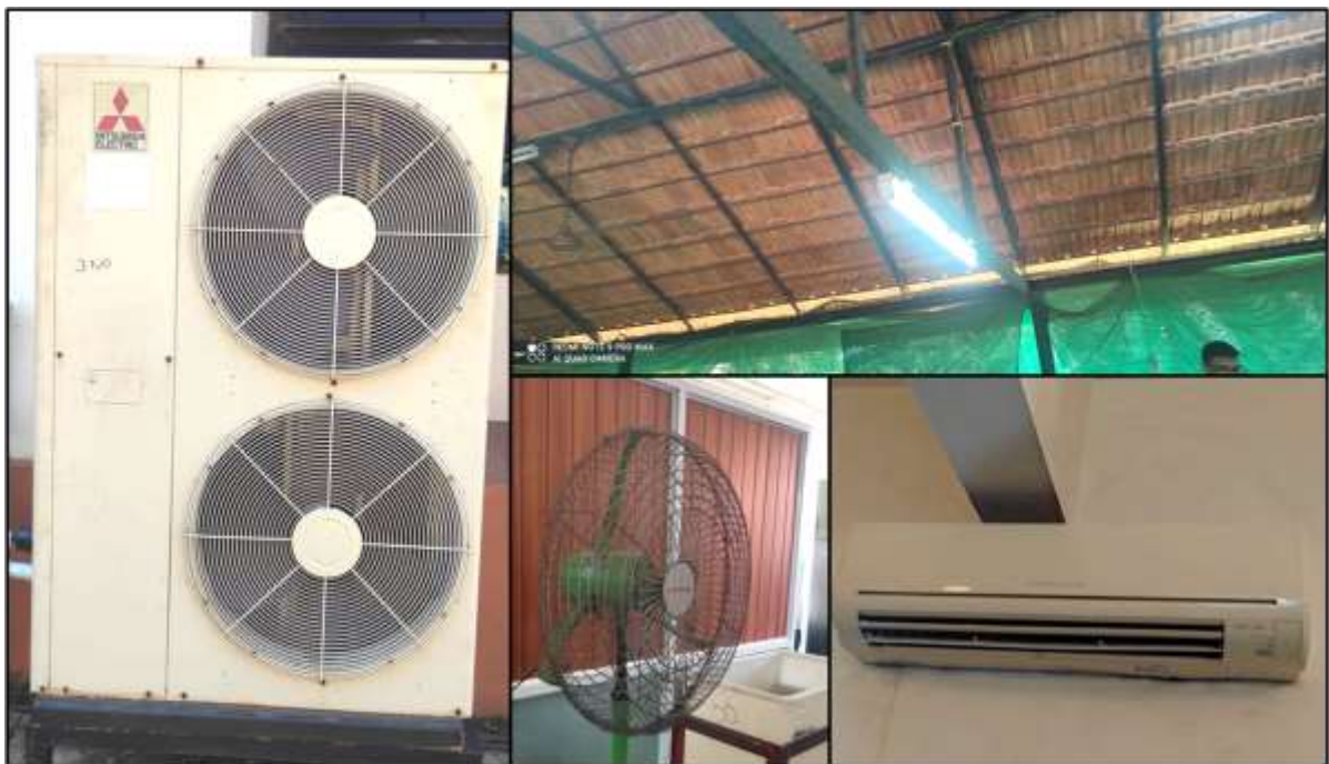
Ventilator, AC, Tube Lights and Fans in Yenepoya (Deemed to be University) Mangalore, Karnataka.
