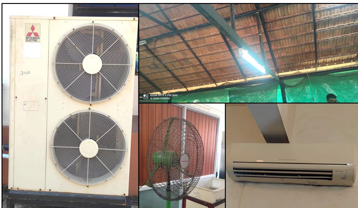
Ventilator, AC, Tube Lights and Fans in Yenepoya (Deemed to be University) Mangalore, Karnataka.
