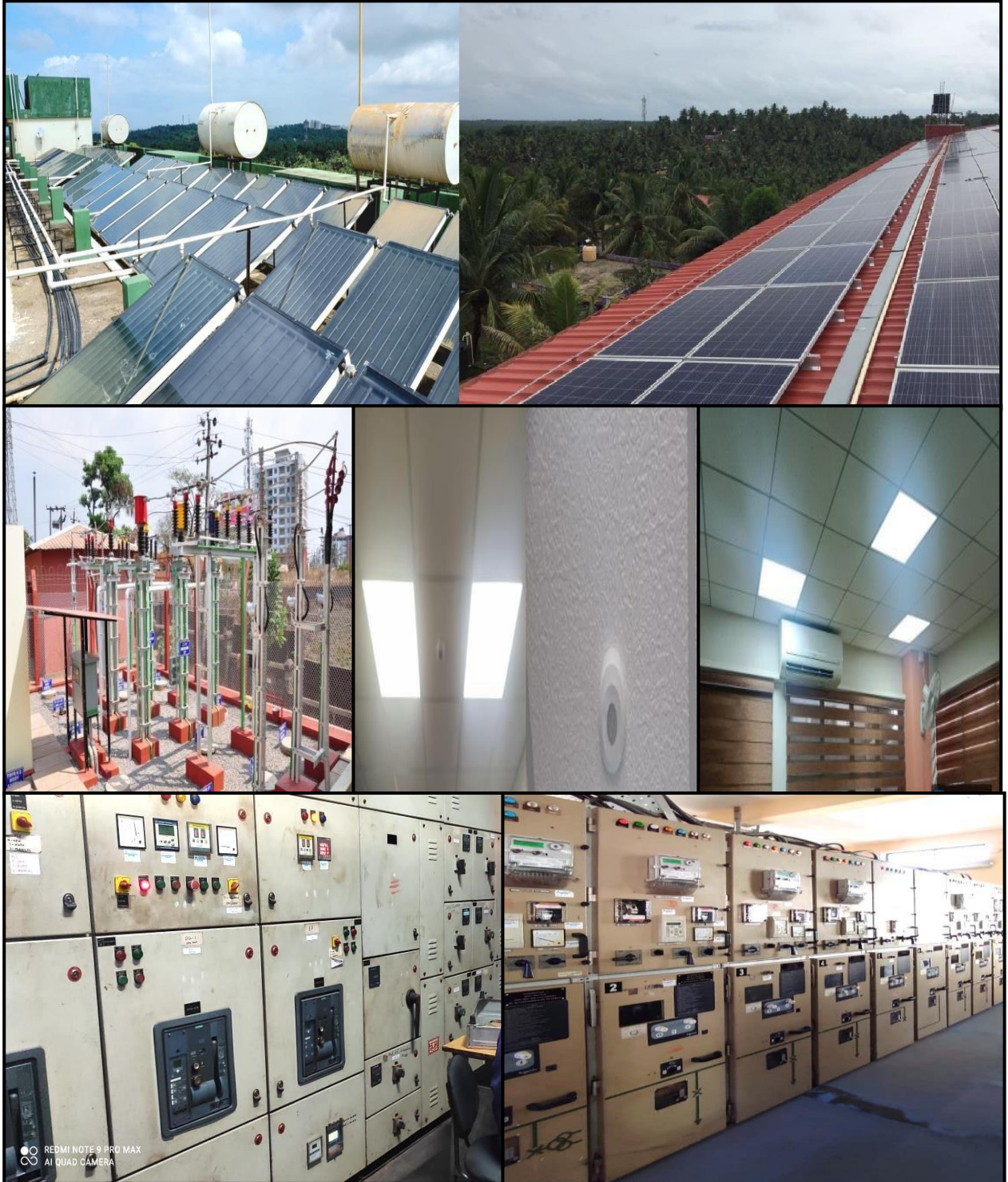
Energy Conservation and Management Activities at Yenepoya (Deemed to be University), Mangalore, Karnataka
