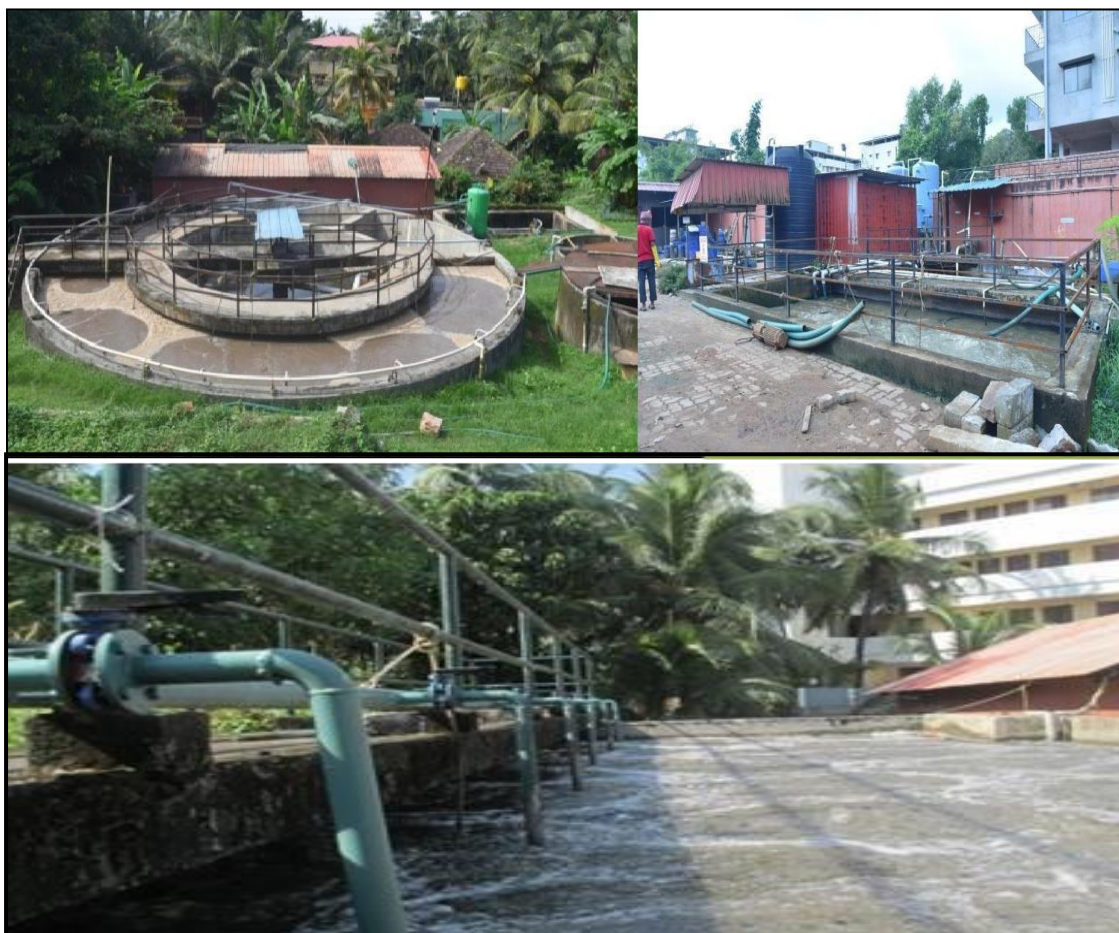
Sewage Treatment Plant (STP) Unit in Yenepoya (Deemed to be University), Mangalore, Karnataka
