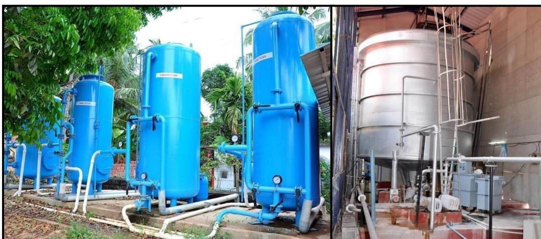
Water Treatment plant and Effluent treatment plant in Yenepoya (Deemed to be University), Mangalore, Karnataka
