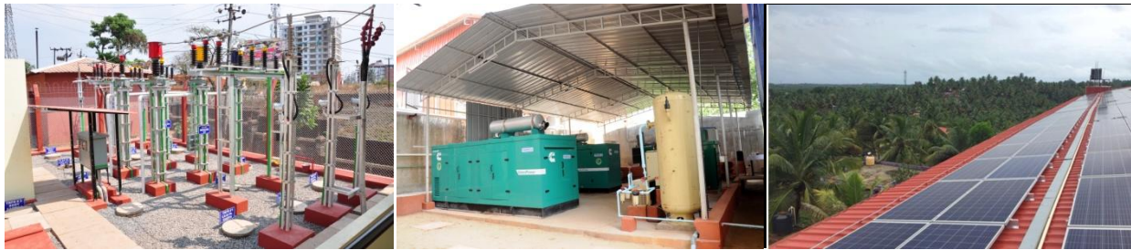
Fig 10. Power station, Diesel Generators and Solar panels
