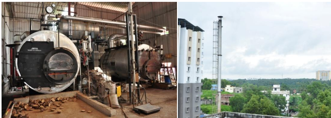
Fig 11. Boiler and Chimney
