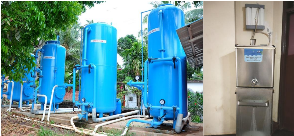
Fig 1: Water treatment plant and Aquaguard
